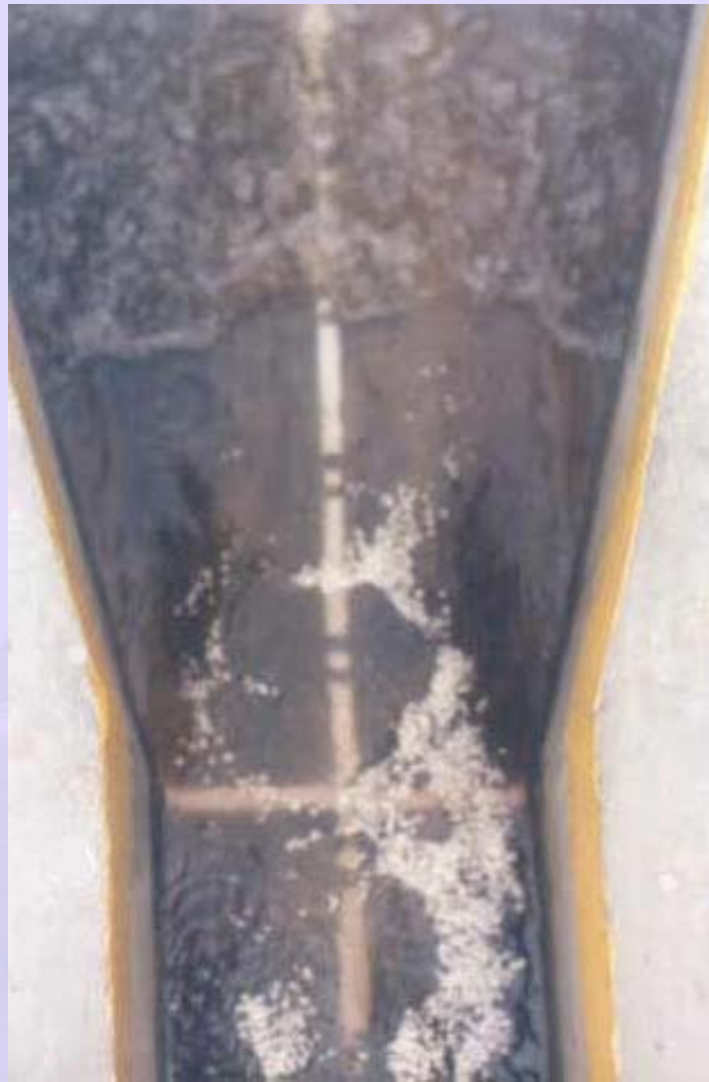
Jump in gradual expansion - looking downstream
